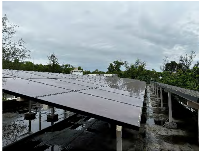
21.5kWp Solar Power plant
